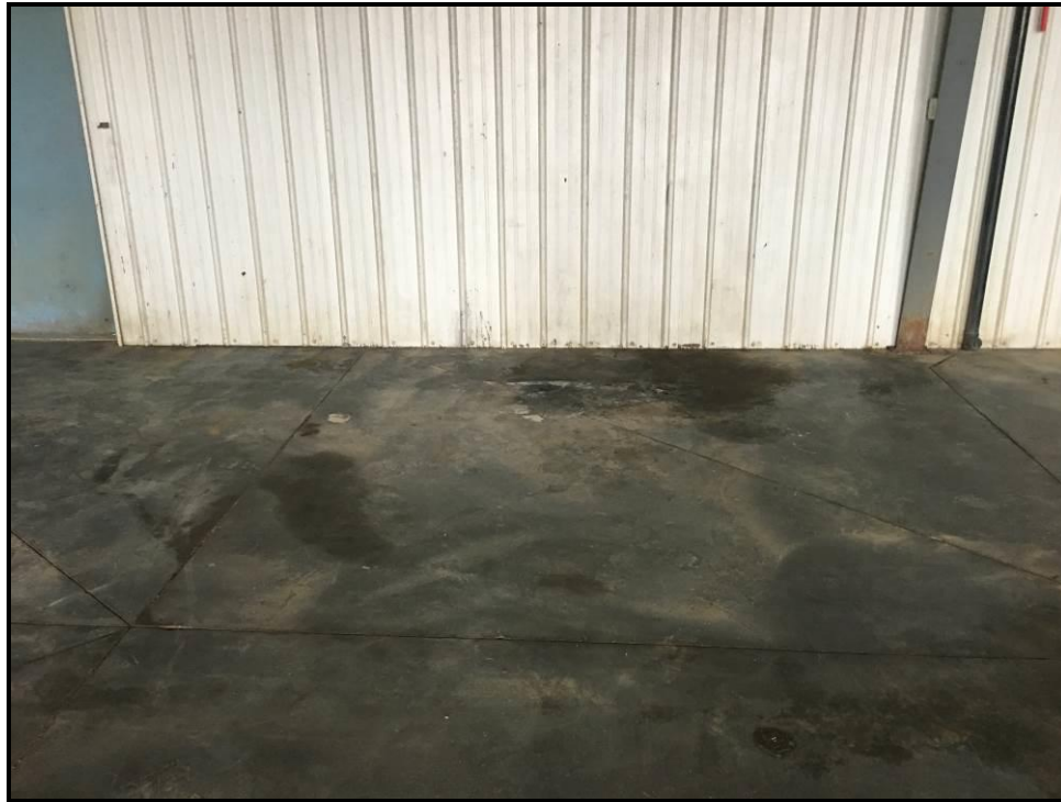
Photograph 3: Surficial staining in the north corner of the shop (September 10, 2018).
