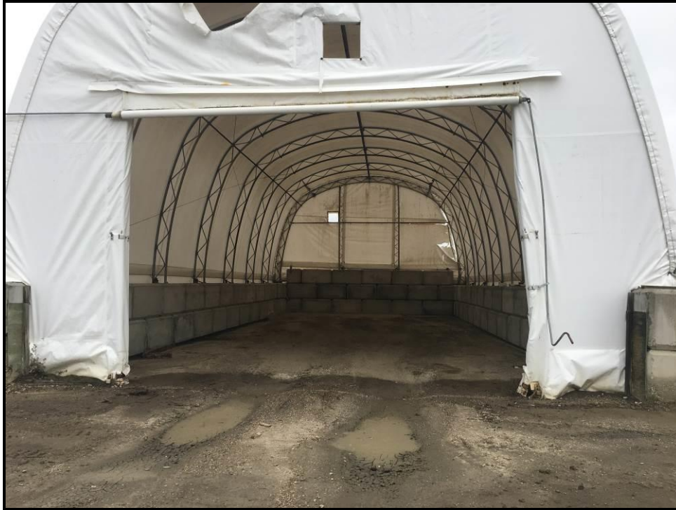
Photograph 5: One of the two empty Quonsets on the Property, formerly utilized for rig mat storage (September 10, 2018).
