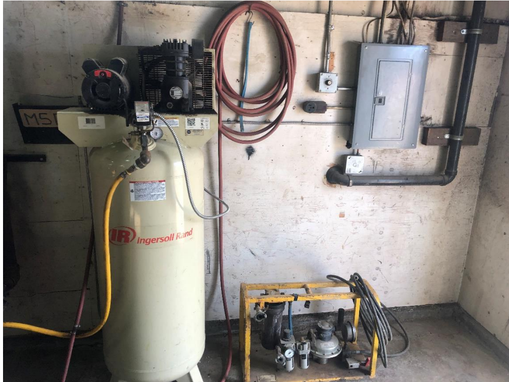
FIGURE 5: MAIN SHOP UTILITY ROOM
