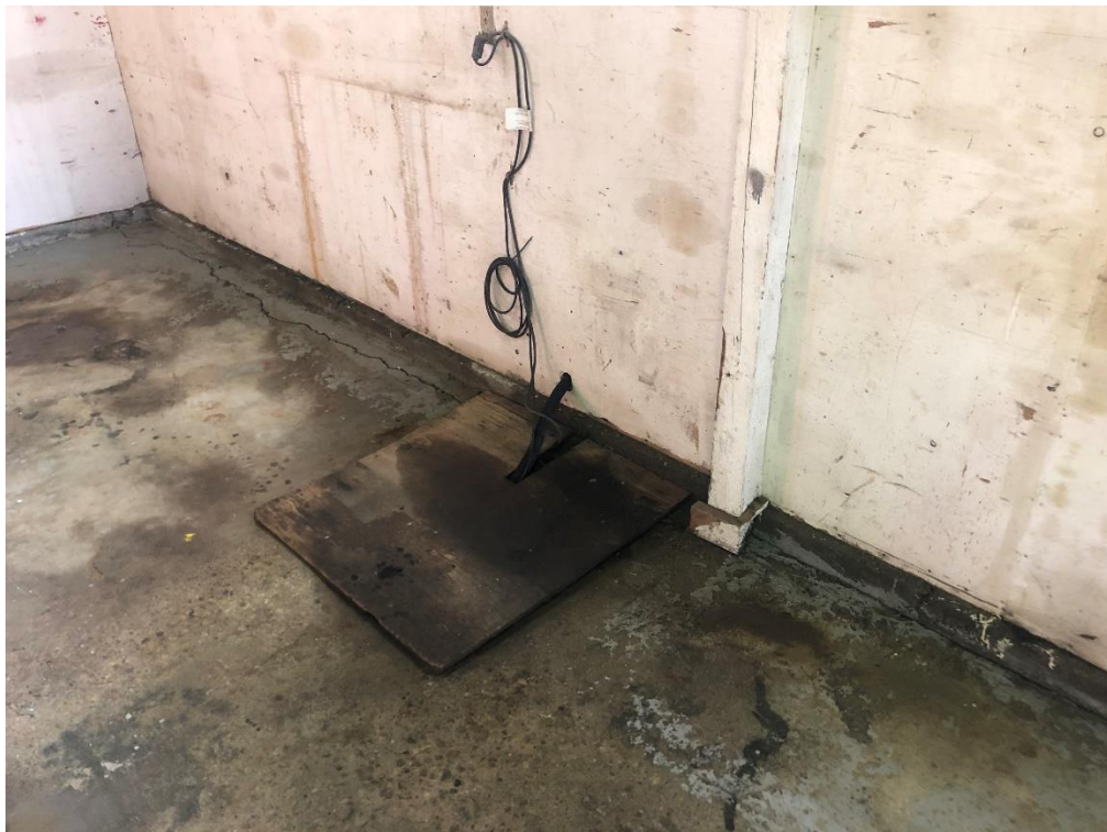
FIGURE 4: SUMP AND DISCHARGE PUMP IN MAIN SHOP
