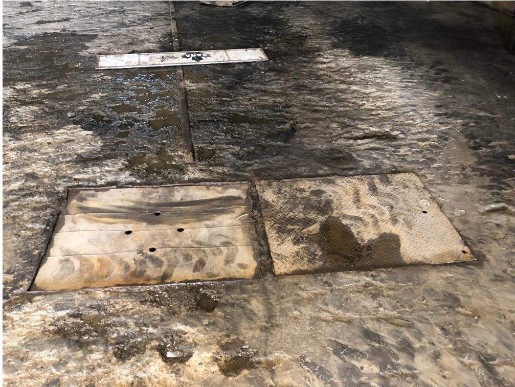
FIGURE 9: OIL/GRIT SEPARATOR IN SECOND SHOP
