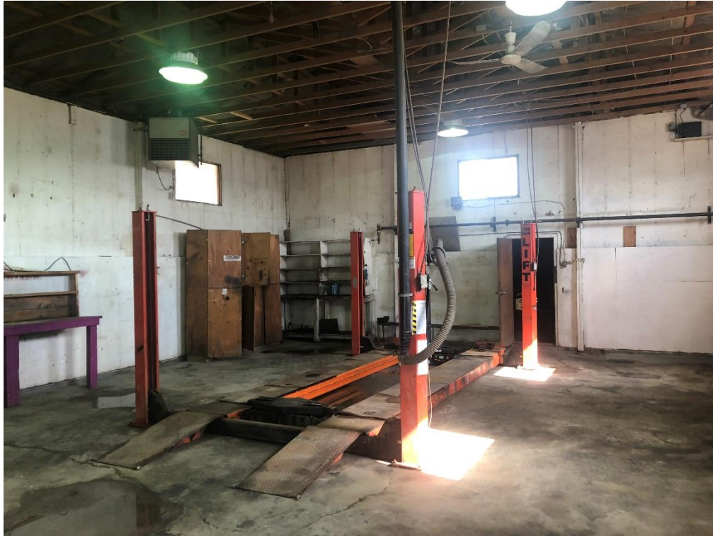
FIGURE 3: VEHICLE HOIST IN MAIN SHOP
