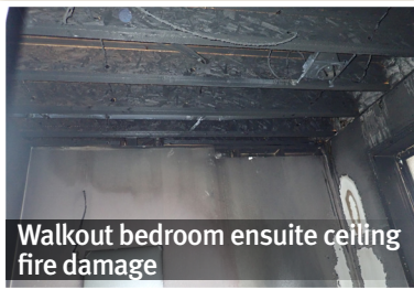
Walkout bedroom – fire damage
