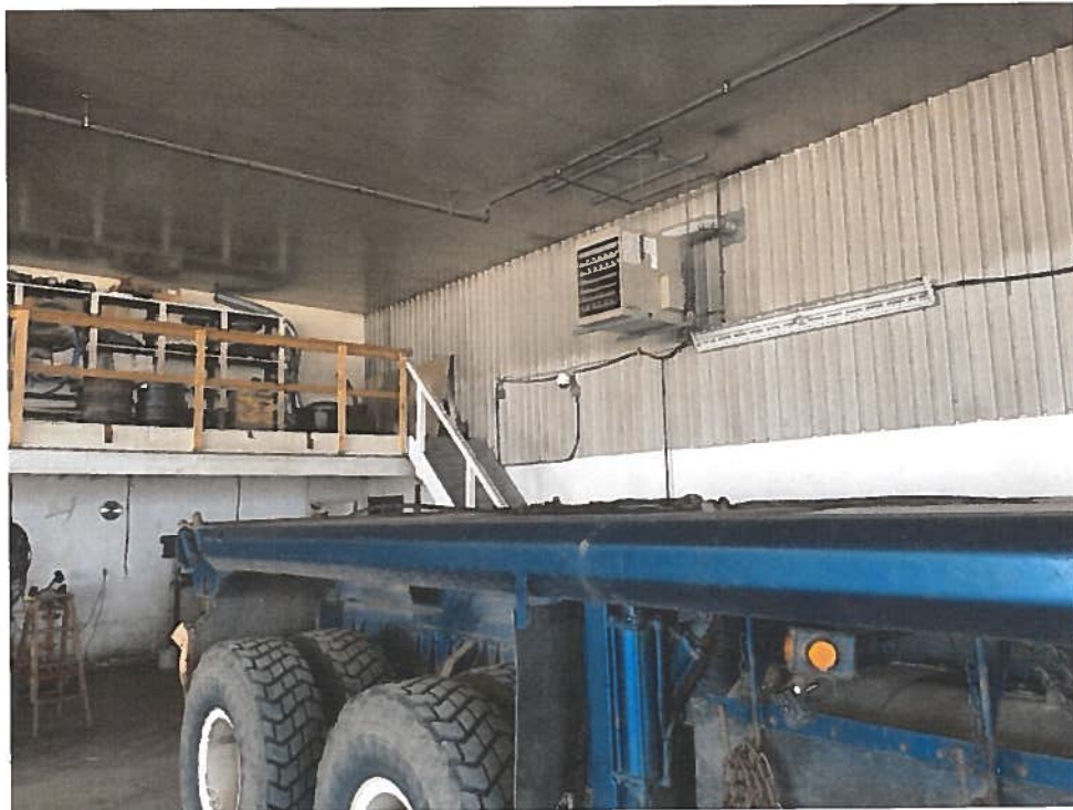
FIGURE 13: SHOP HEATING UNITS
