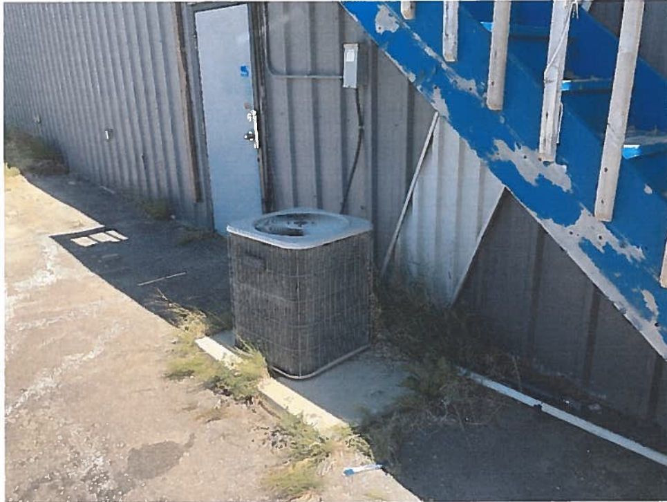
FIGURE 8: EXTERIOR AC UNIT
