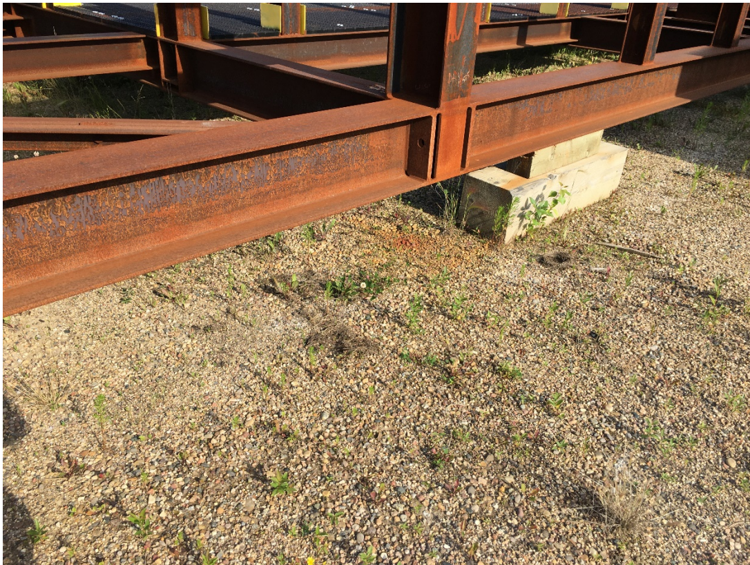
Photo 4: Rust staining beneath the module frames..
