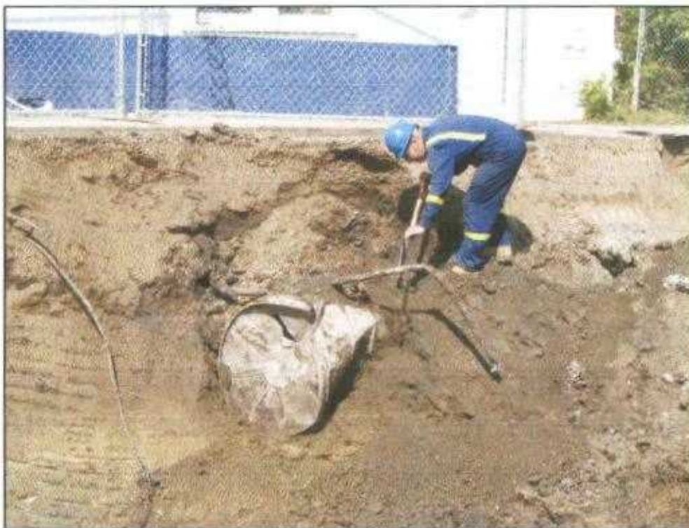
Photograph 4: Site # 5720 – Exposing unexpected UST.
