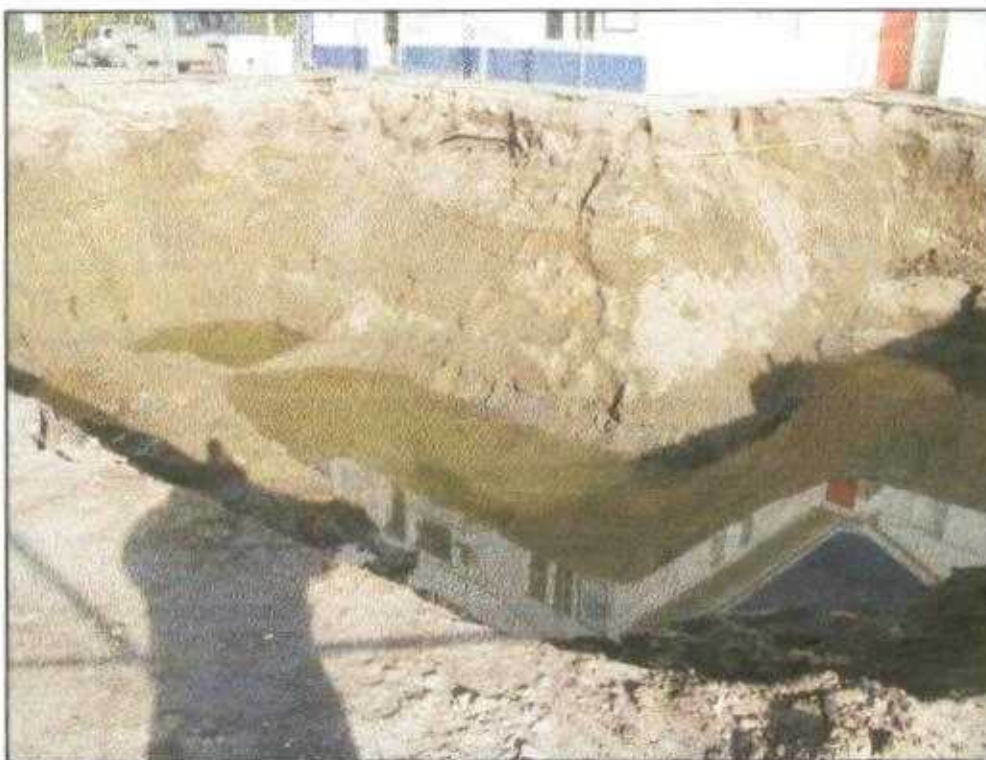
Photograph 5: Site # 5720 – Exposed west, and north excavation walls, note water in the excavation.
