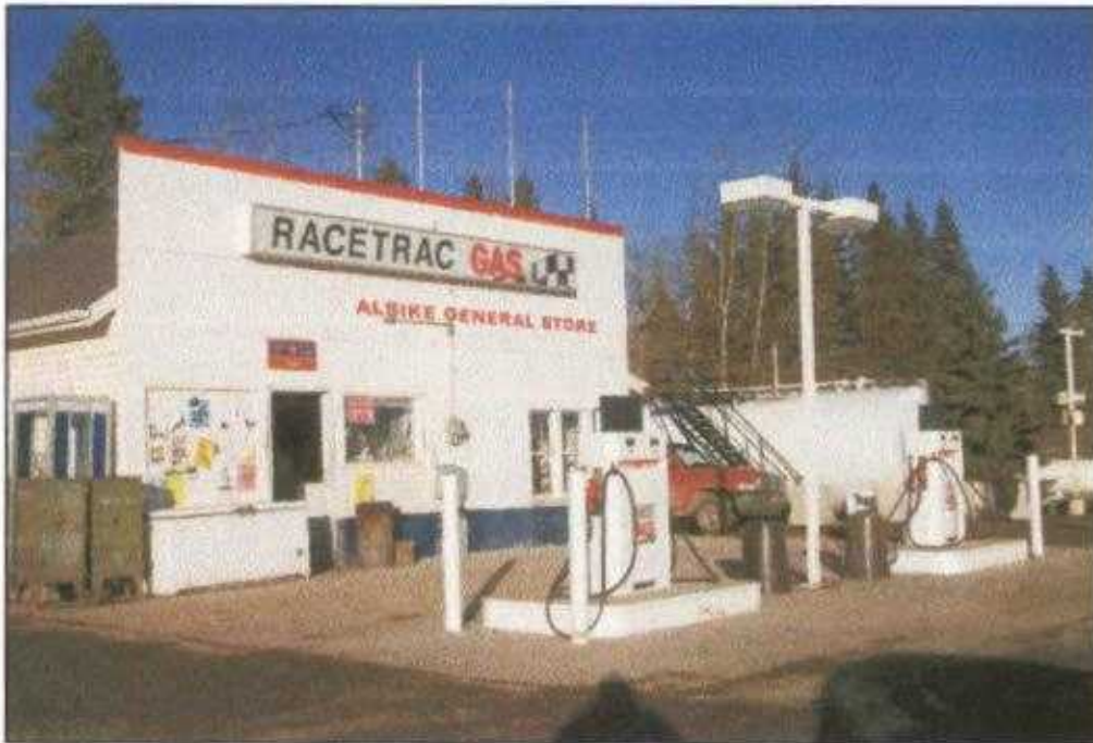
Photograph 9: Site # 5720 – View looking northeast after installation of concrete pad and pump islands.
