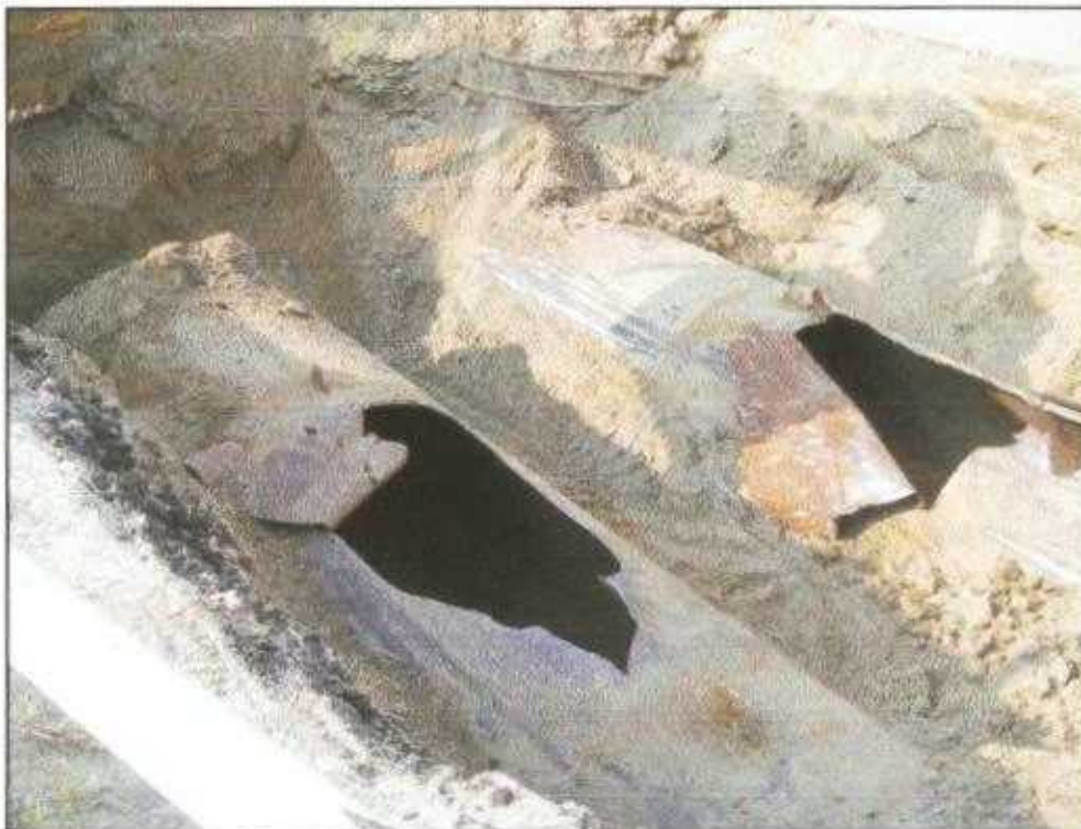
Photograph 3: Site # 5720 – Two exposed and inerted underground storage tanks.
