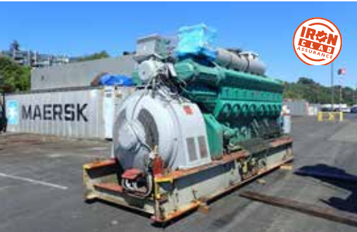
1 of 3 – EMD A11 1000 KW – Located in Seattle, WA
