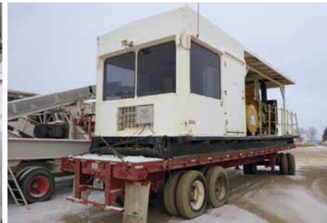
Caterpillar 570 KW w/Control House
