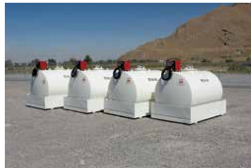
Large Quantity of Unused Tanks
