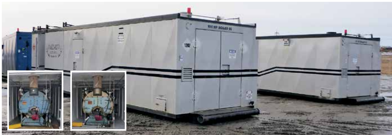
Williams & Davis 777 100 HP Boiler & Williams & Davis 777 80 HP Boiler
