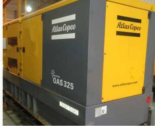
QTY OF ATLAS COPCO GENERATOR SETS
