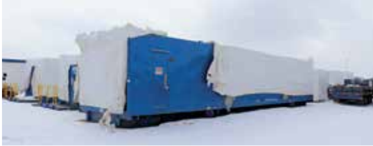
2014 NOV Power Distribution House
